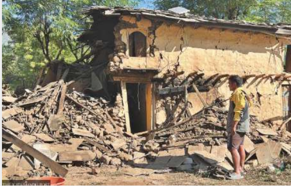
A man inspects the remains of a house destroyed by the quake in Aathbiskot-14 on Saturday.
