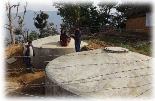
Tanks constructed with project support, Lekhgaun Drinking Water Scheme, Lekhgaun, Surkhet
