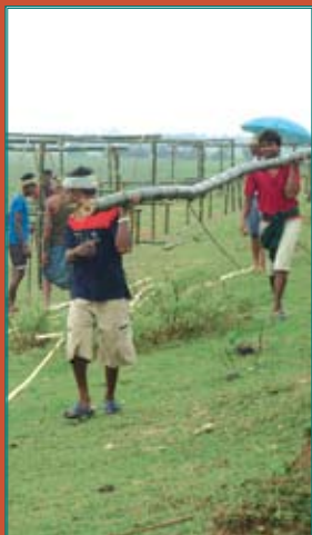
Constructing rehabilitation center as a response mechanism for flood, Saptari Photo: Eco-Nepal
